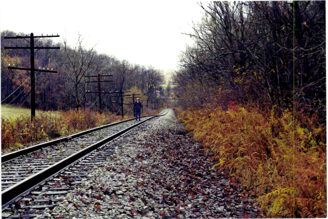
Figure 26. Subsidence is visible along a railroad, Washington County. The upper photo shows the five feet of new ballast necessary here to restore railroad function after longwall mining. The lower photo shows that subsidence has continued since repairs were made to the roadbed.
