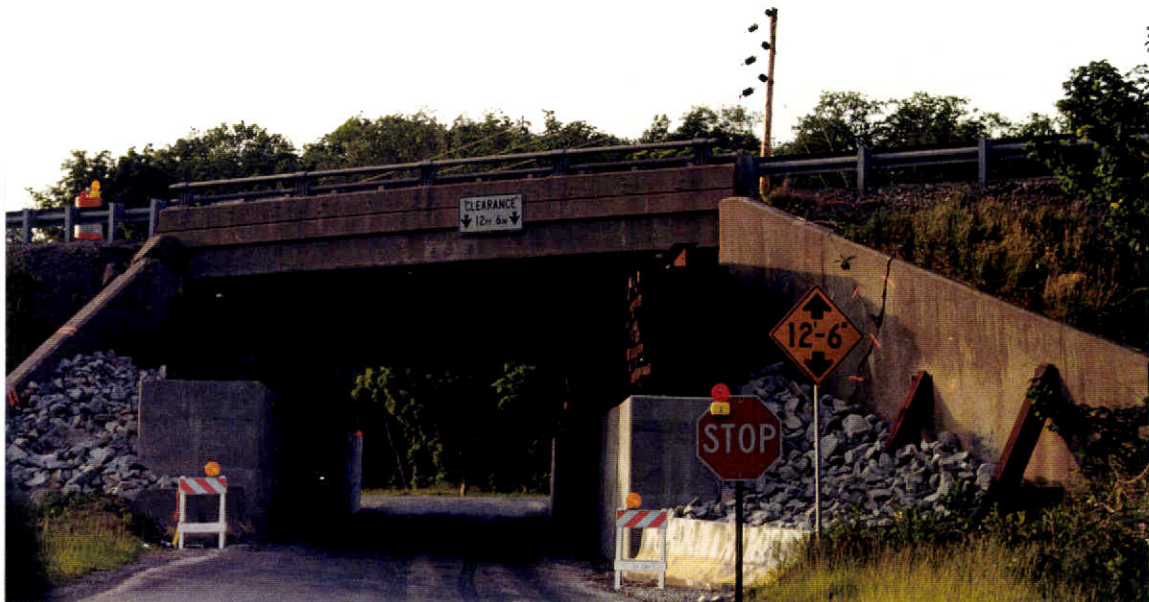
Figure 15. Subsidence damage to Interstate 70 following longwall mining, Washington County. The bridge opening can no longer accommodate two lanes of traffic. Wetland damage is not so obvious to the casual observer.
